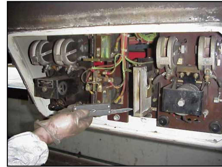
In fuse box linings outside of car, on side of the train 17534 Flash guards Chrysotile
