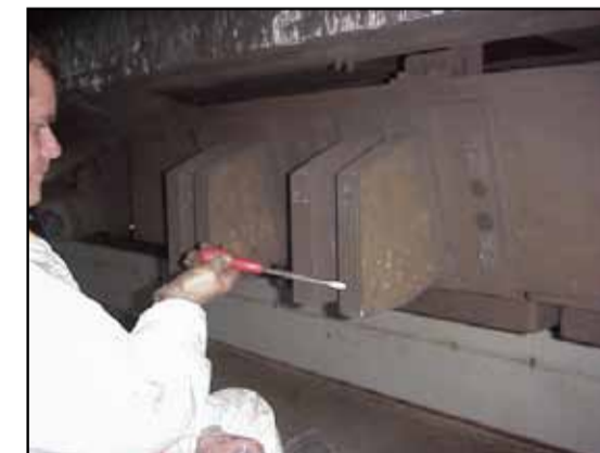
Outside equipment case No 2, outside car on side of train 7534 Flash guards Chrysotile
