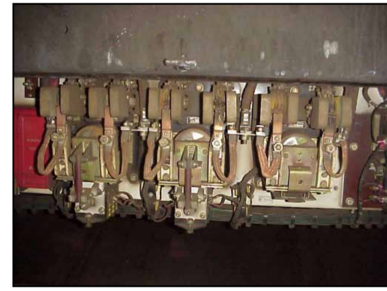
In fuse box linings outside of car, on side of the train 7534 Flash guards Chrysotile
