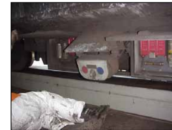
In fuse box linings outside of car, on side of the train 7534 Board. Chrysotile
