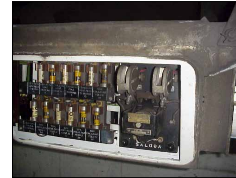
In heater contact case outside of car, on side of train 17534 Flash guards. Chrysotile
