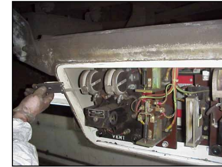
In field failure case, outside of car on side of the train 17534 Flash guards Chrysotile
