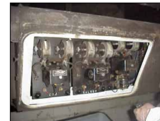
In equipment case No 9, outside car on side of train 7534 Flash guards Amosite & Chrysotile
