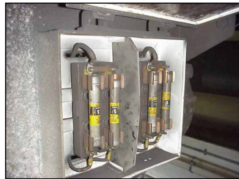
In equipment case No 13, Outside car on side of train Flash guards Chrysotile
