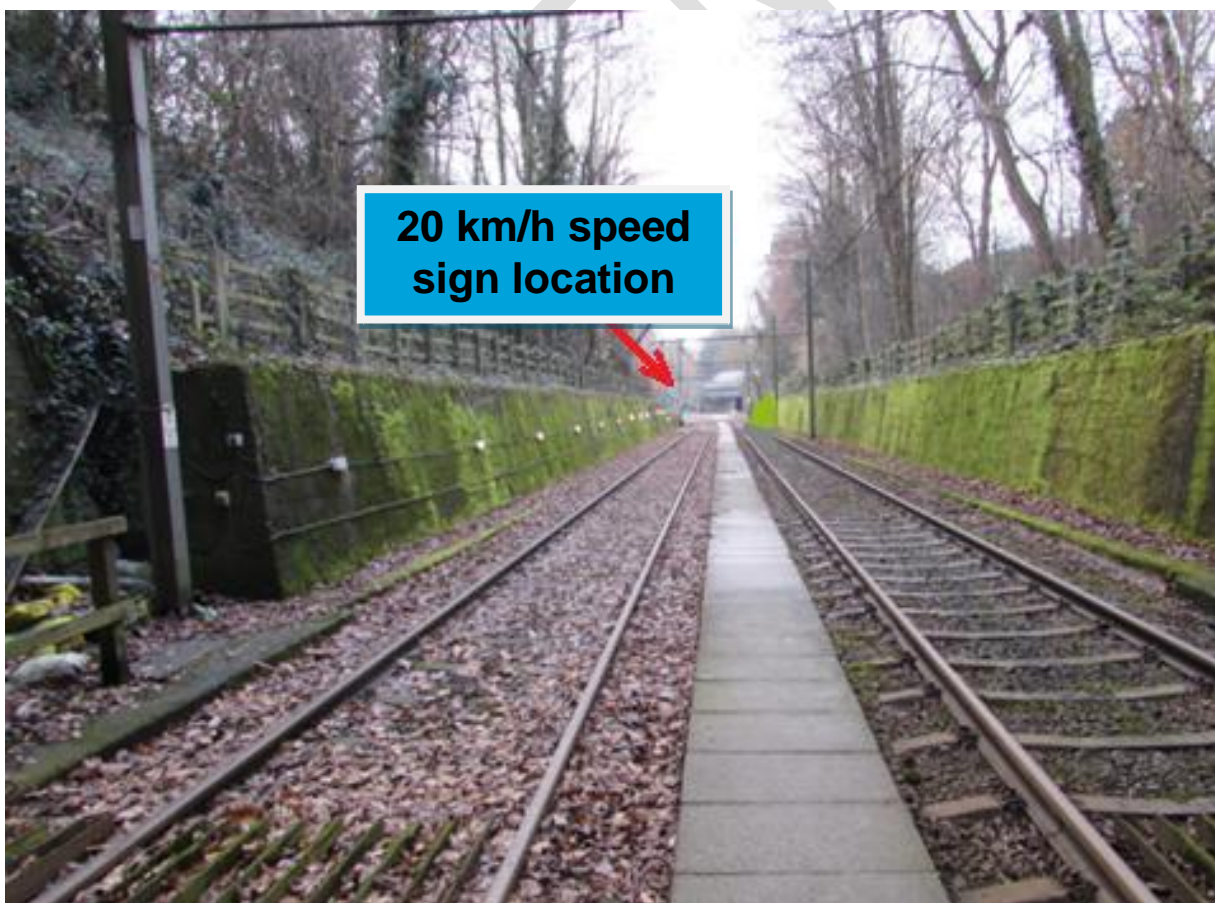
Figure 6 - 20km/h board on exit from Woodside tunnel (photo taken around 85m from the start of the curve)
