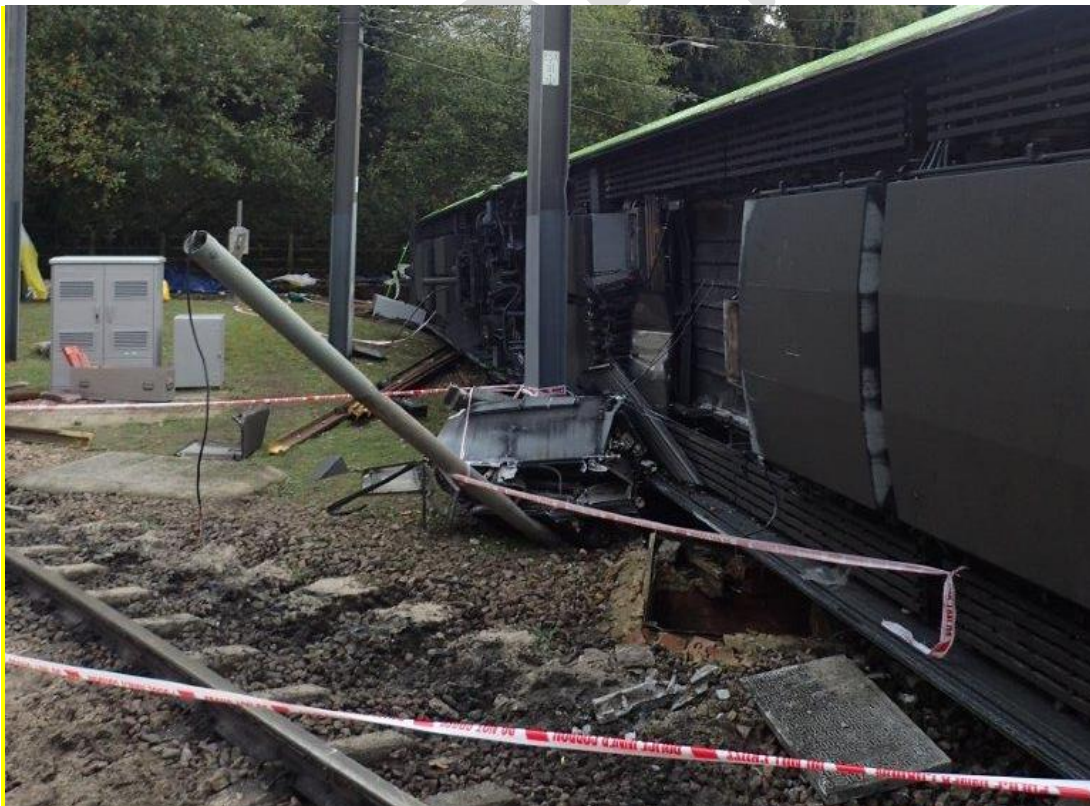
Figure 2 - Tram 2551 roof against infrastructure
