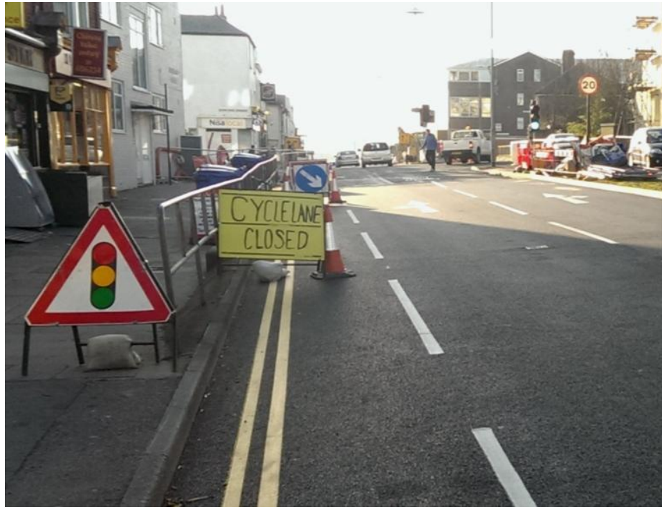
Poor treatment at road works
