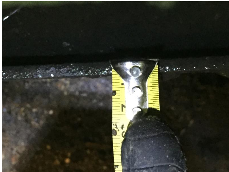
Photo 1 – Original fixing plate thickness – 5mm
