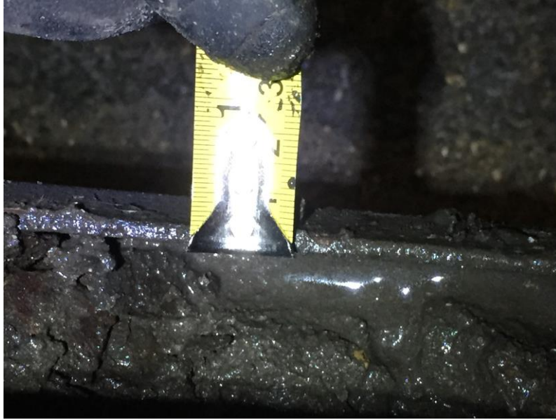
Photo 2 – Reduction in fixing plate thickness – 2mm
