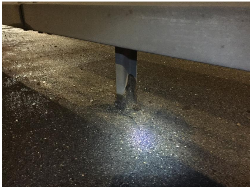
Photo 3 – Corrosion on posts
