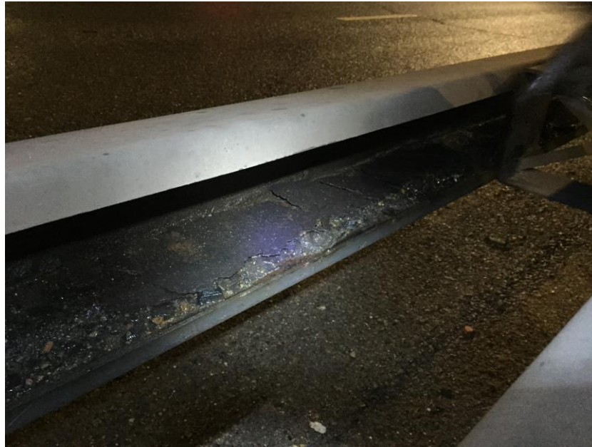
Photo 5 – Beam Inner Face Exfoliation
