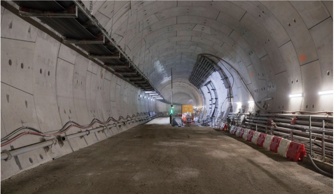
The images show the base of the new tunnel's road surface in place (photo: Riverlinx)
