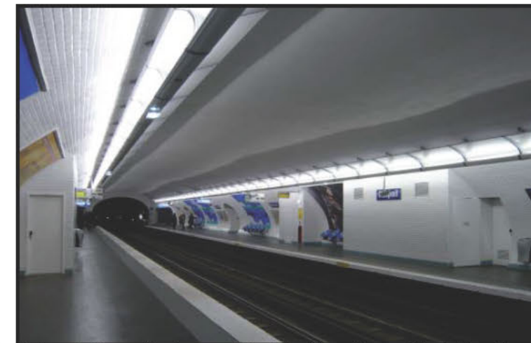
Ceiling of station without ceramic tiles to limit the reflection of the lighting fitting. Light is reflected and diffused by the surface.
