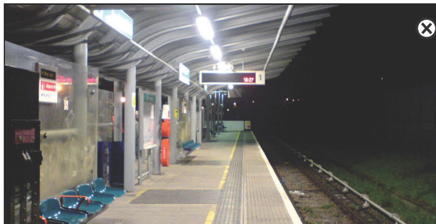
Purely functional lighting using surface mounted luminaires with no optical control. No feature lighting or lighting for wayfinding provides for an unattractive space.
