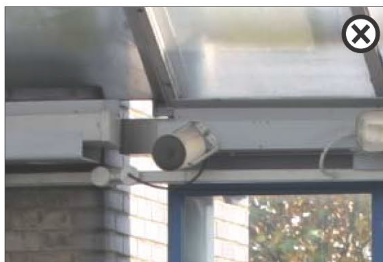
PA Speakers at Crossharbour station platform
