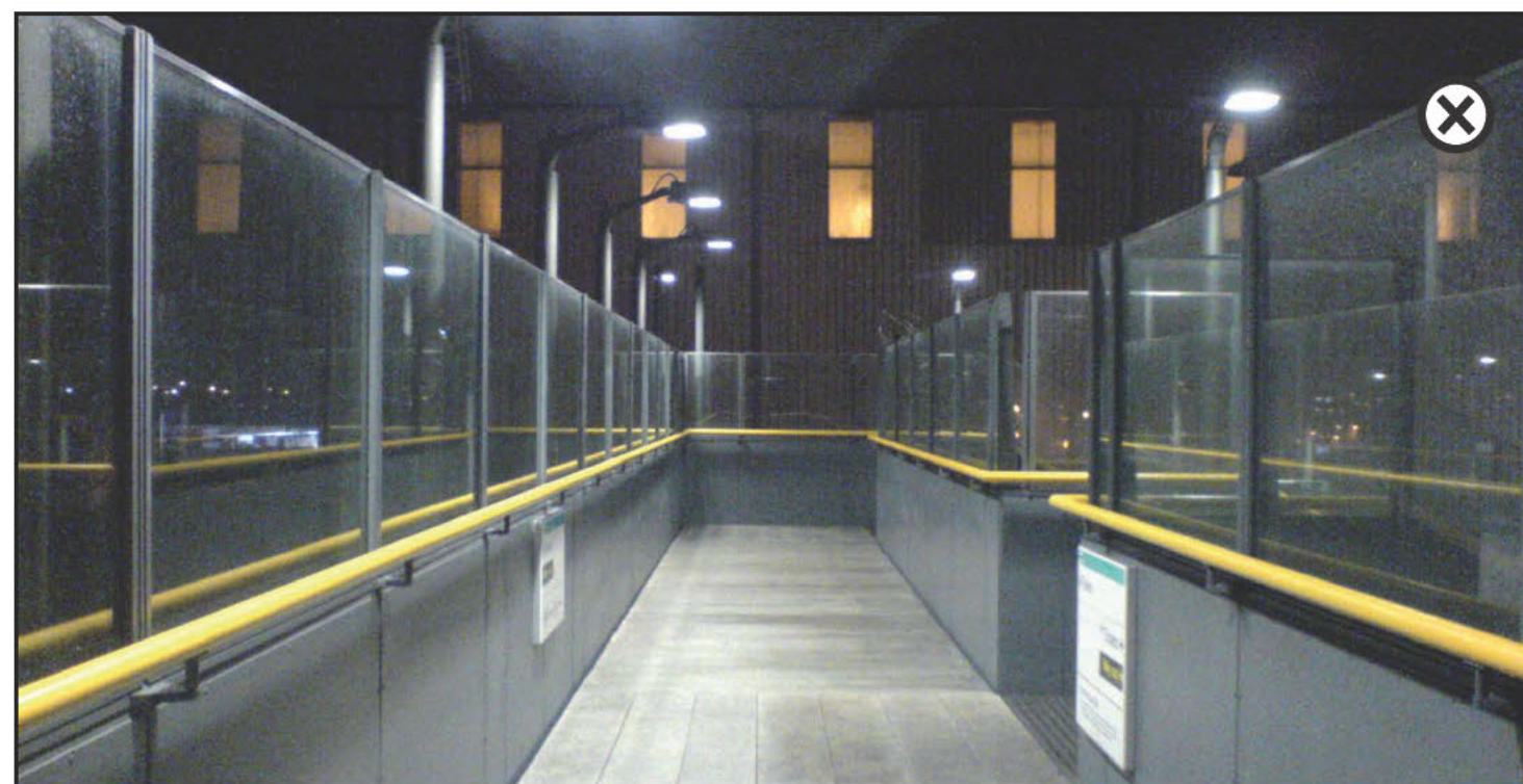
Lighting columns are not integrated into structure and provide visual clutter both in the short and long views to the bridge.
