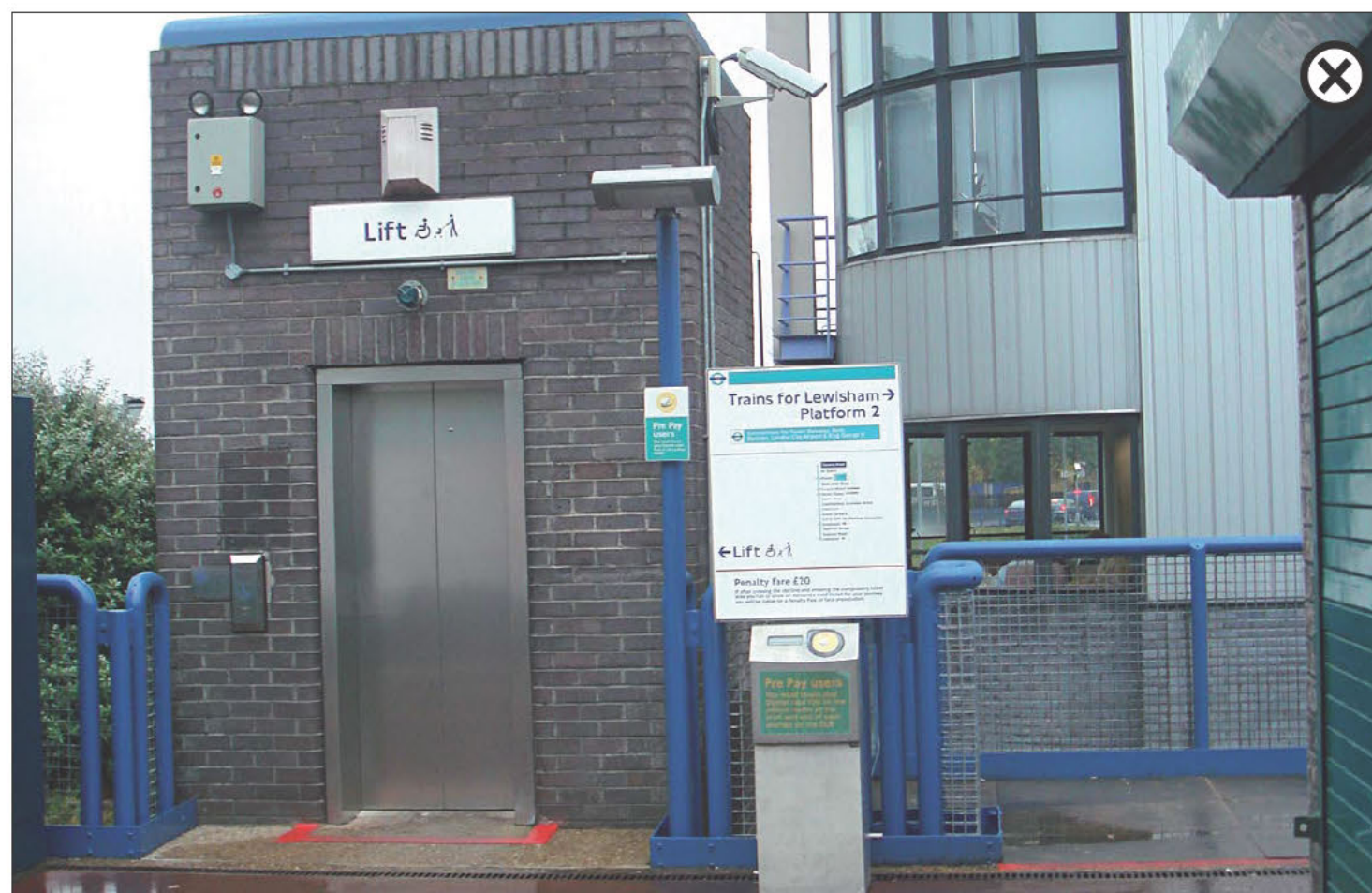
Devons Road station lift has an untidy appearance with conduit, alarm and other items fixed to the exterior.
