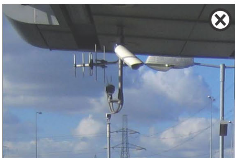
CCTV cameras at Canning Town station
