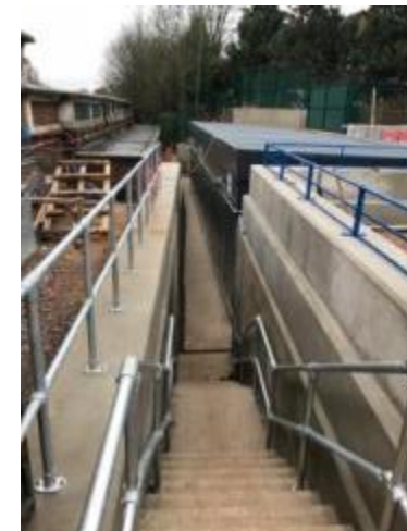
Extensive excavation at Ealing Common to protect heritage of the existing station building
