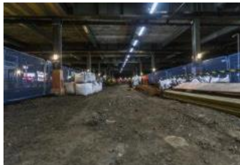
Piling beneath an undercroft of Sainsbury's, all deliveries by Engineering Trains at Triangle sidings
