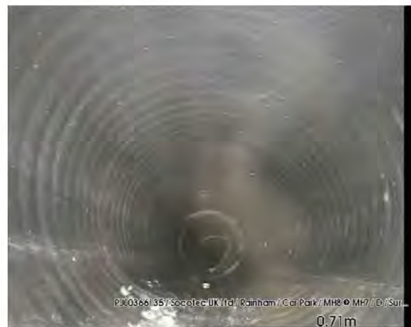
200317_1336C-Survey.jpg, 00:00:20, 0.71 m Deformed drain or sewer, 10% %
