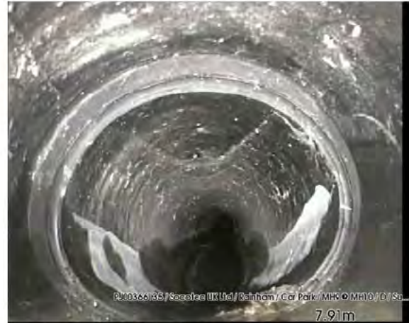
200317_1442A-Survey.jpg, 00:01:29, 7.91 m Deformed drain or sewer, 20% %
