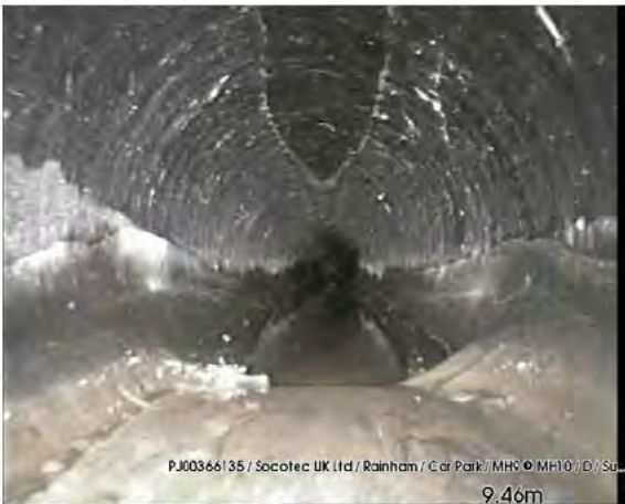
200317_1442B-Survey.jpg, 00:02:05, 9.46 m Deformed drain or sewer, 10% %
