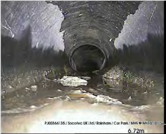
200317_1441B-Survey.jpg, 00:00:52, 6.72 m Settled deposits, coarse, 10% % cross-sectional area loss
