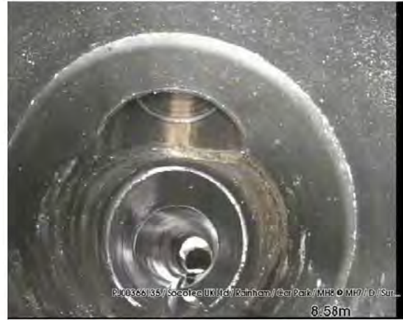
200317_1338A-Survey.jpg, 00:00:54, 8.58 m Junction, at 12 o'clock, diameter: 100 mm
