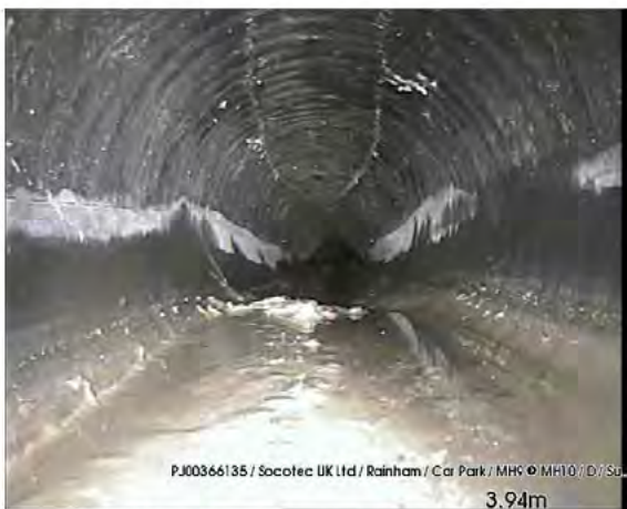
200317_1440E-Survey.jpg, 00:00:32, 3.94 m Settled deposits, fine, 10% % cross-sectional area loss
