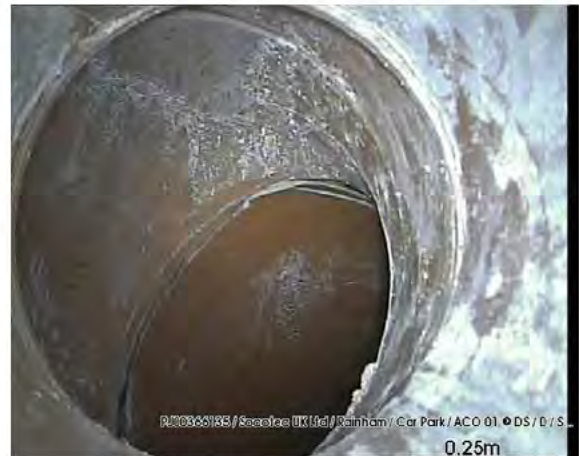
200317_1238A-Survey.jpg, 00:00:14, 0.25 m Line deviates right
