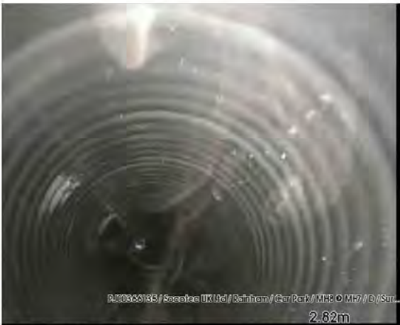
200317_1337B-Survey.jpg, 00:00:34, 2.86 m Line deviates down
