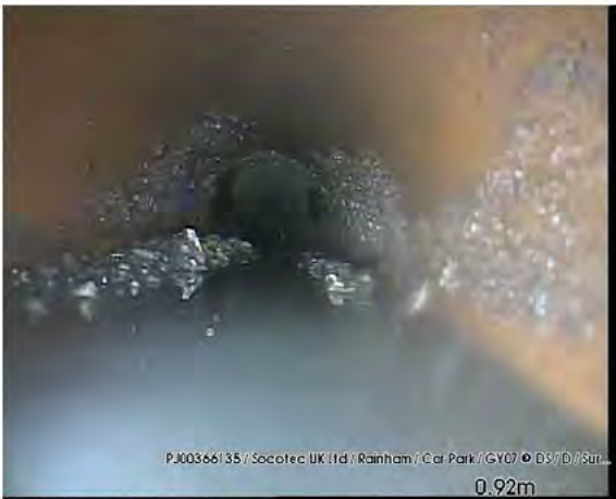
200318_1432E-Survey.jpg, 00:00:14, 0.92 m Settled deposits, fine, 10% % cross-sectional area loss
