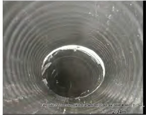
200317_1337A-Survey.jpg, 00:00:30, 2.34 m Deformed drain or sewer, 40% %
