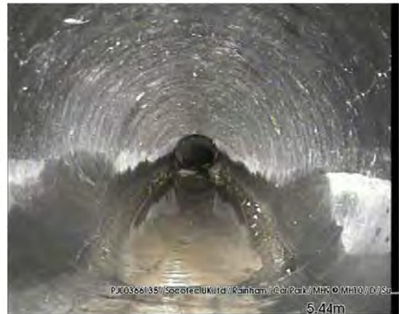
200317_1441A-Survey.jpg, 00:00:41, 5.44 m Line deviates down
