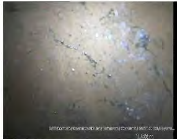
200318_1411B-Survey.jpg, 00:00:23, 1.83 m Finish node type, other special chamber, reference number: DS, reached
