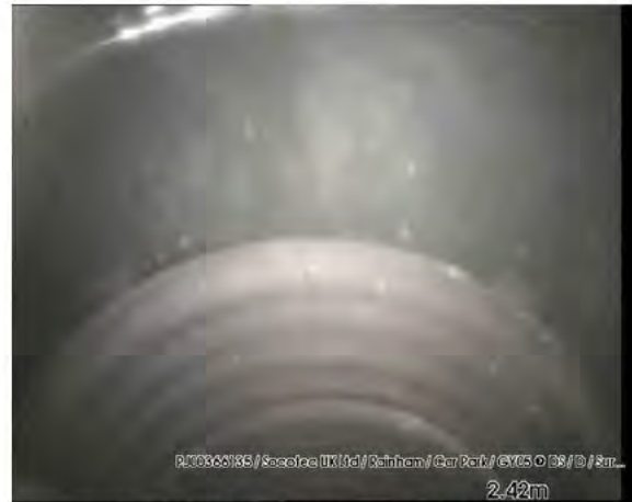
200318_1203A-Survey.jpg, 00:00:27, 2.42 m Line deviates down
