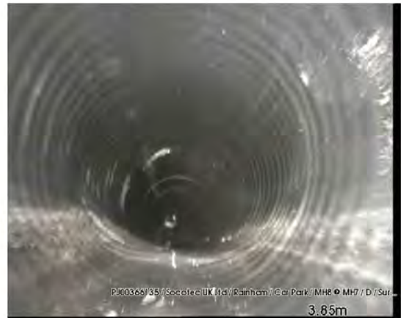
200317_1337C-Survey.jpg, 00:00:38, 3.85 m Deformed drain or sewer, 30% %
