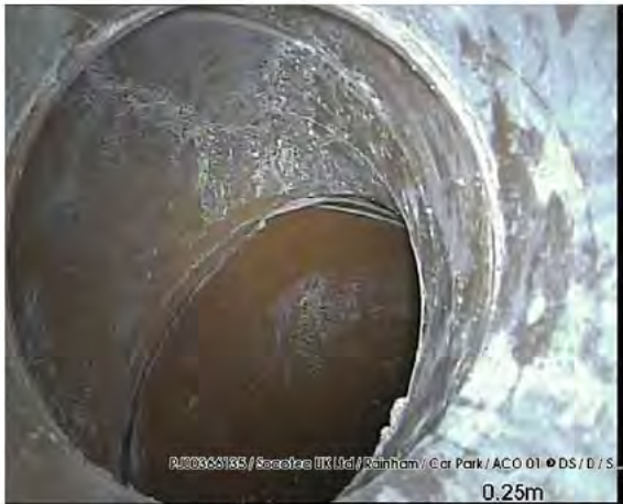
200317_1238B-Survey.jpg, 00:00:16, 0.25 m Line deviates down
