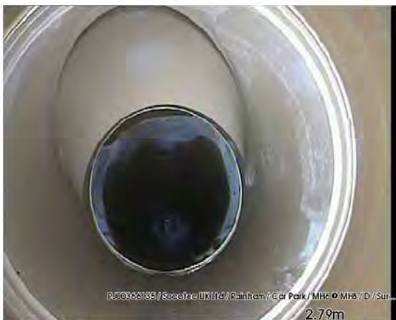
200317_1232B-Survey.jpg, 00:00:11, 2.79 m Junction, at 11 o'clock, diameter: 150 mm
