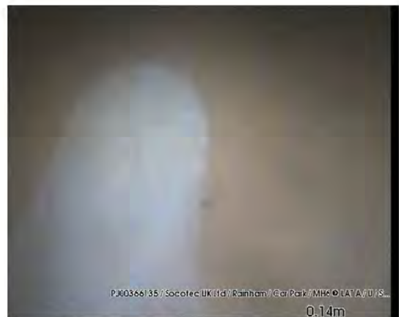
200317_1202F-Survey.jpg, 00:00:12, 0.14 m Line deviates up
