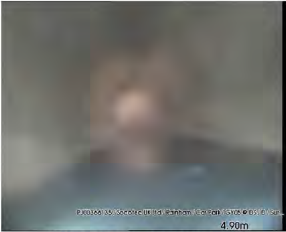
200318_1203D-Survey.jpg, 00:00:51, 4.90 m Finish node type, other special chamber, reference number: DS, reached
