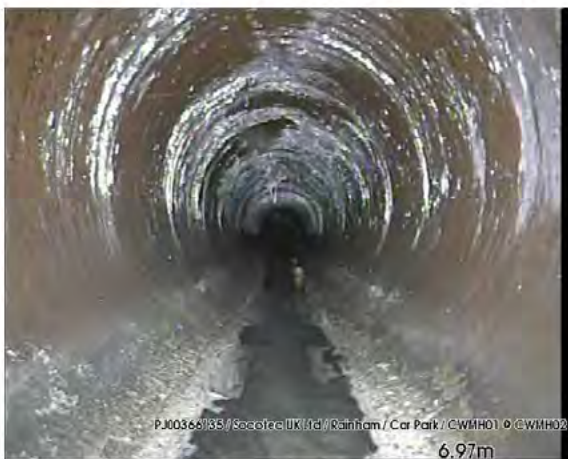
200317_1457A-Survey.jpg, 00:00:35, 6.97 m Line deviates down
