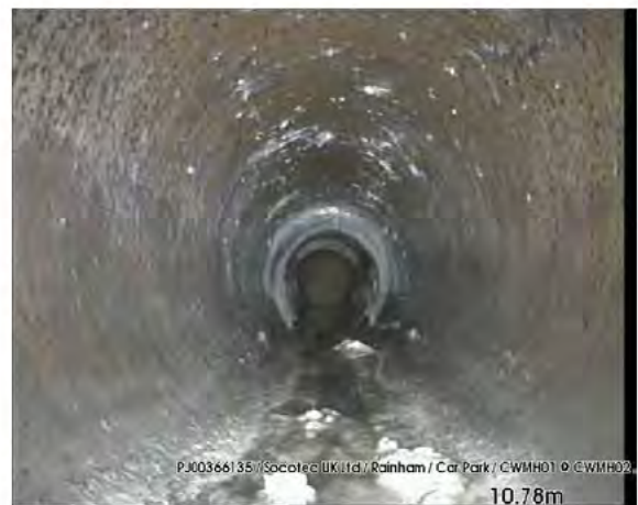
200317_1457B-Survey.jpg, 00:00:51, 10.78 m Line deviates down
