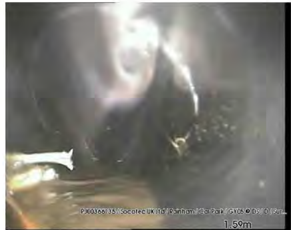
200318_1202F-Survey.jpg, 00:00:20, 1.59 m Deformed drain or sewer, 10% %
