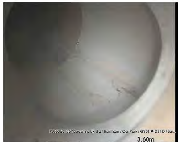
200317_1205F-Survey.jpg, 00:00:21, 3.60 m Finish node type, other special chamber, reference number: DS, REACHED
