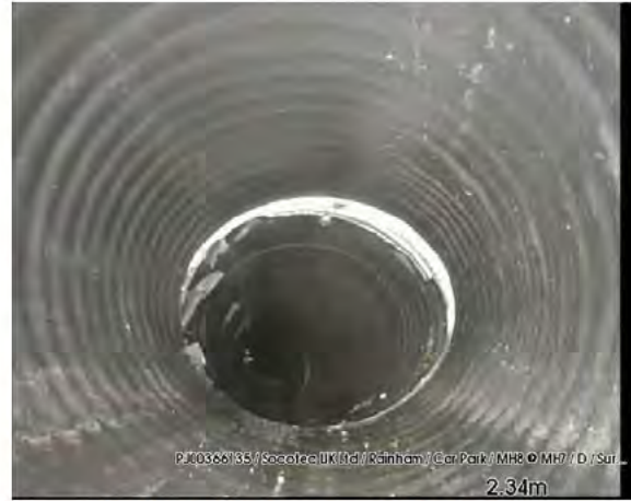
200317_1337A-Survey.jpg, 00:00:30, 2.34 m Deformed drain or sewer, 40% %
