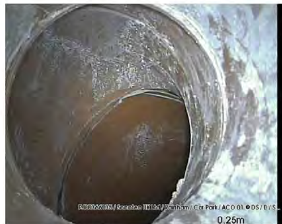
200317_1238A-Survey.jpg, 00:00:14, 0.25 m Line deviates right
