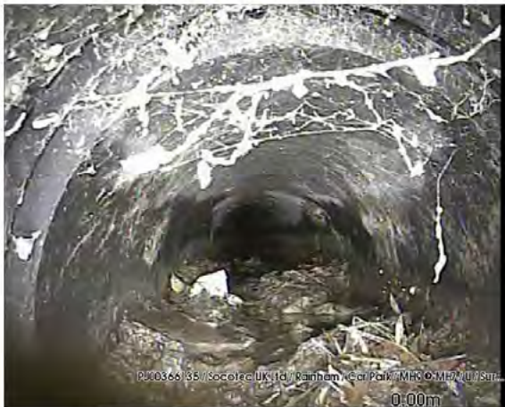
200317_1436A-Survey.jpg, 00:00:09, 0.00 m Settled deposits, fine, 40% % cross-sectional area loss
