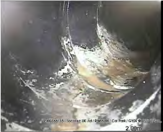
200318_1418E-Survey.jpg, 00:00:22, 2.00 m Line deviates right
