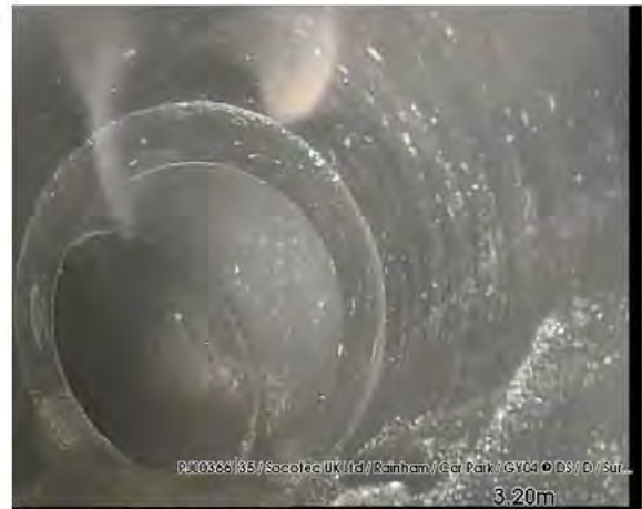
200318_1145B-Survey.jpg, 00:00:24, 3.20 m Line deviates left
