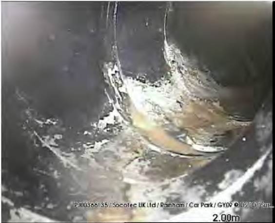
200318_1418E-Survey.jpg, 00:00:22, 2.00 m Line deviates right
