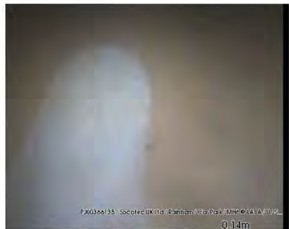
200317_1202F-Survey.jpg, 00:00:12, 0.14 m Line deviates up
