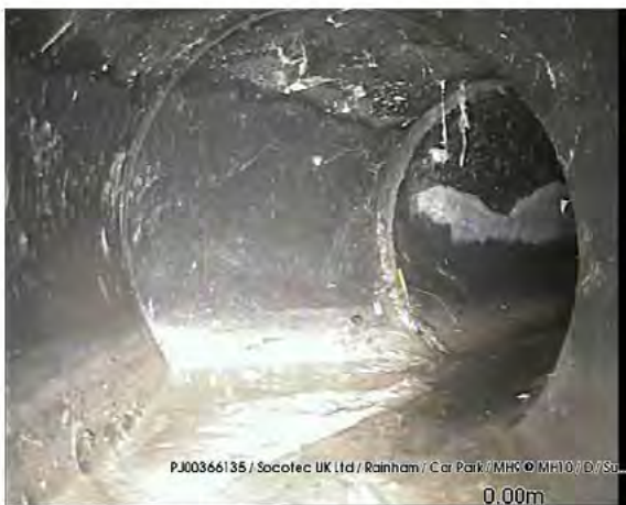
200317_1440A-Survey.jpg, 00:00:04, 0.00 m Line deviates right
