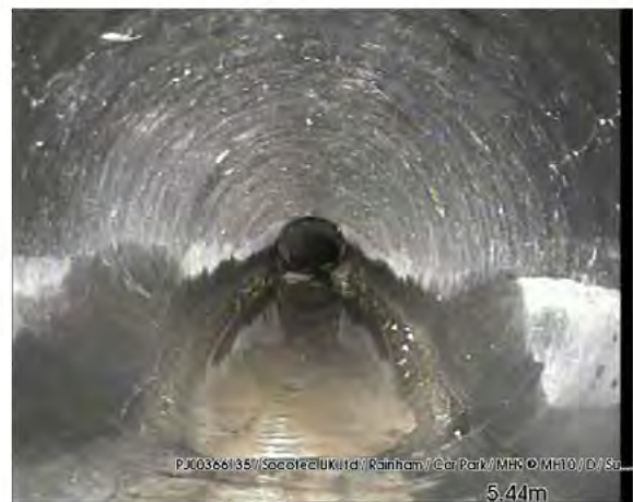
200317_1441A-Survey.jpg, 00:00:41, 5.44 m Line deviates down
