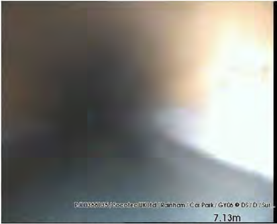
200318_1355B-Survey.jpg, 00:00:42, 7.13 m Settled deposits, fine, 10% % cross-sectional area loss
