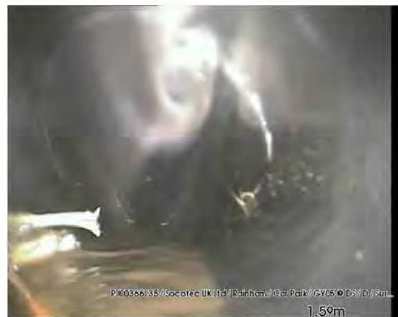
200318_1202F-Survey.jpg, 00:00:20, 1.59 m Deformed drain or sewer, 10% %
