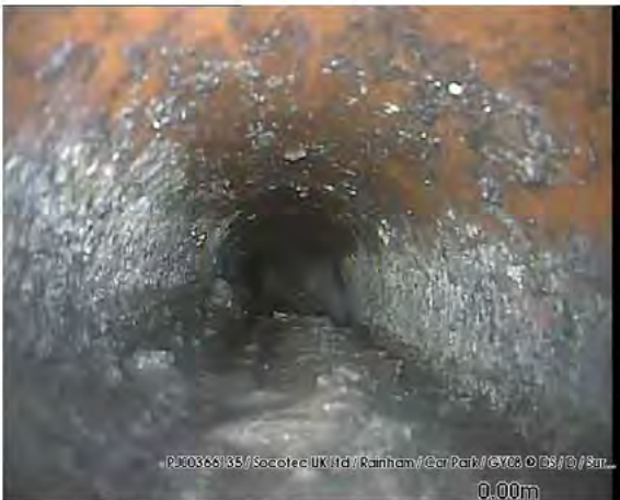
200318_1411A-Survey.jpg, 00:00:04, 0.00 m Settled deposits, fine, 10% % cross-sectional area loss
