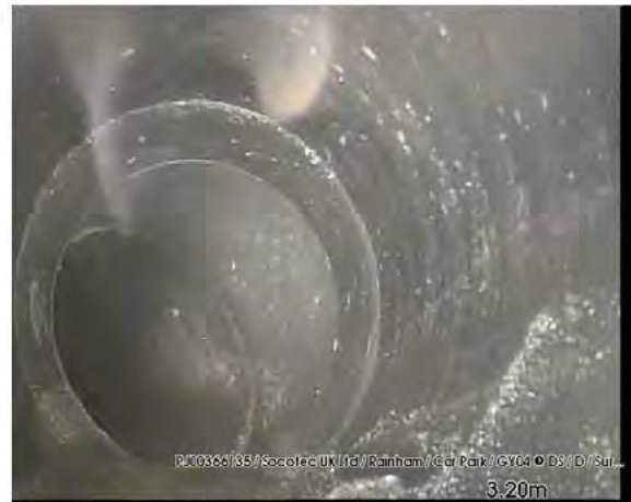
200318_1145B-Survey.jpg, 00:00:24, 3.20 m Line deviates left
