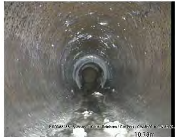
200317_1457B-Survey.jpg, 00:00:51, 10.78 m Line deviates down
