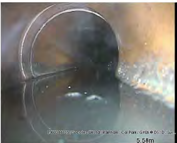
200318_1354E-Survey.jpg, 00:00:28, 5.58 m Line deviates right
