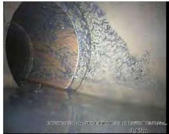
200318_1433A-Survey.jpg, 00:00:39, 3.87 m Finish node type, other special chamber, reference number: DS, reached
