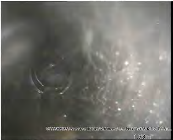
200318_1202G-Survey.jpg, 00:00:22, 1.78 m Line deviates down
