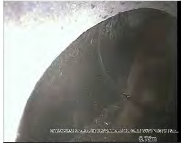
200318_1146A-Survey.jpg, 00:00:41, 5.75 m Finish node type, other special chamber, reference number: DS, reached
