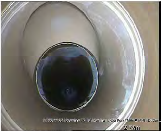
200317_1232B-Survey.jpg, 00:00:11, 2.79 m Junction, at 11 o'clock, diameter: 150 mm
