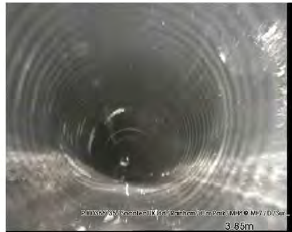
200317_1337C-Survey.jpg, 00:00:38, 3.85 m Deformed drain or sewer, 30% %
