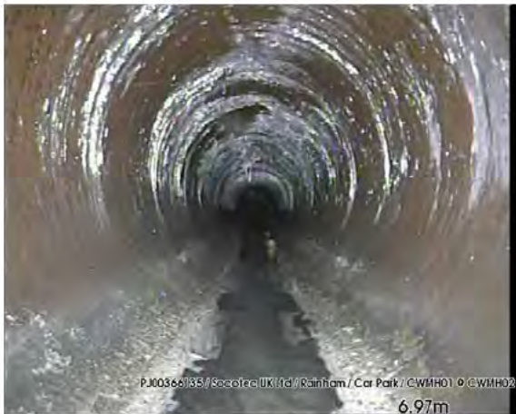
200317_1457A-Survey.jpg, 00:00:35, 6.97 m Line deviates down
