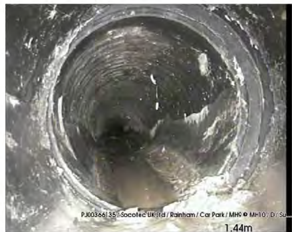
200317_1440B-Survey.jpg, 00:00:15, 1.44 m Line deviates left
