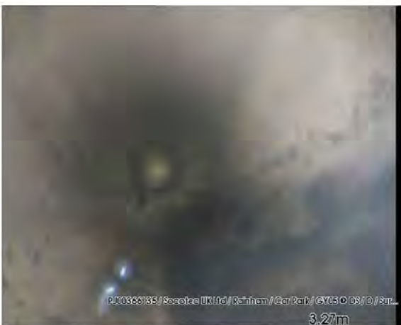
200318_1203B-Survey.jpg, 00:00:33, 3.27 m Material changes Vitrified clay pipe @REM
