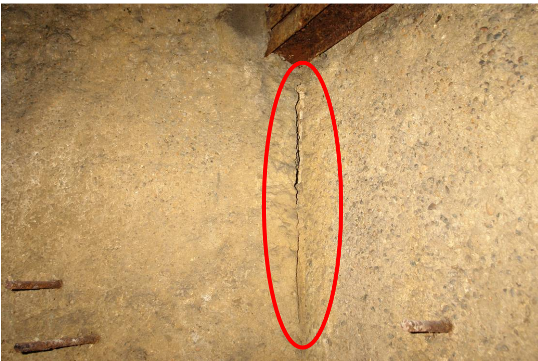
Figure 6 Gap in joint between wall panels
