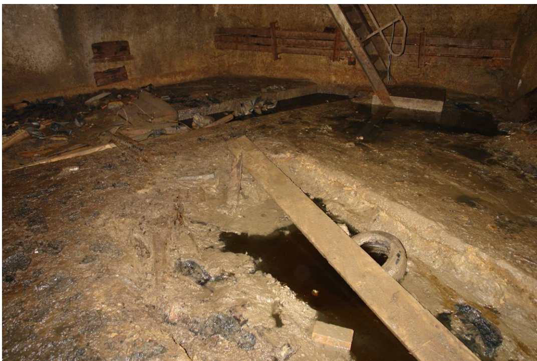
Figure 8 Base slab of shaft covered in mud and debris
