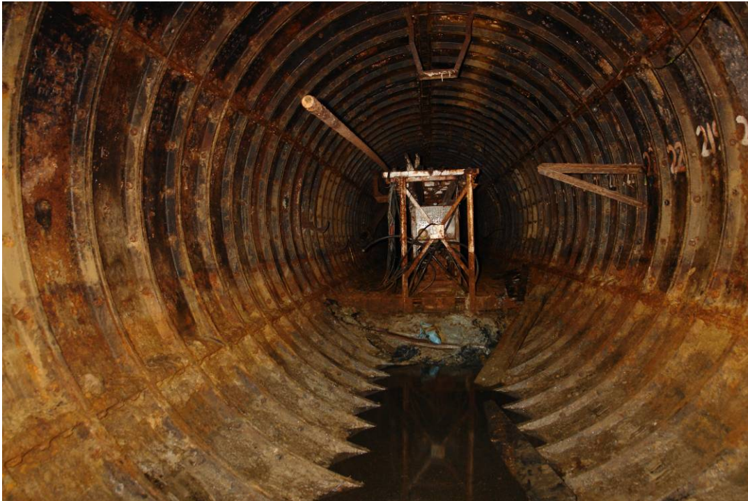
Figure 17 Rear of abandoned tunnelling machine (segment No 230); note water level at approximately 1.5m depth
