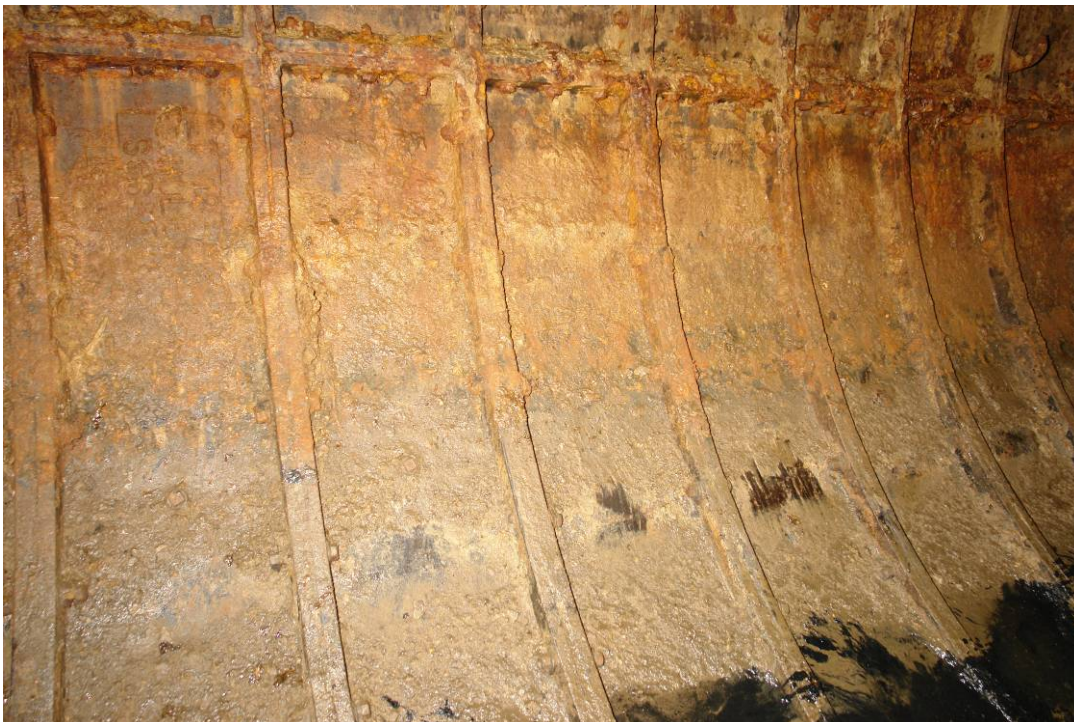
Figure 16 Higher levels of silting towards further end of tunnel (segment No 180)
