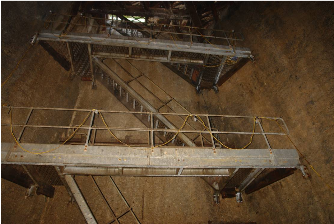
Figure 9 Access stairs and landings in shaft
