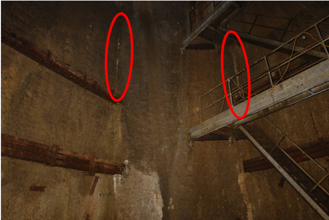
Figure 7 Signs of leakage through joints between walls
