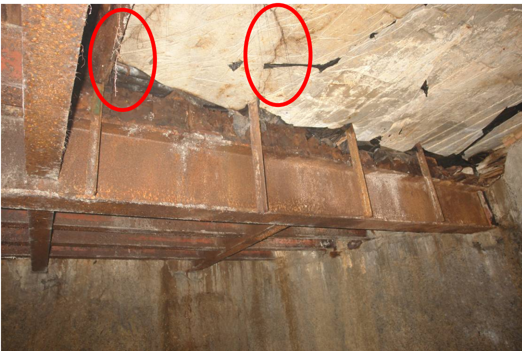
Figure 2 Underside of capping slab, showing some root penetration through crack
