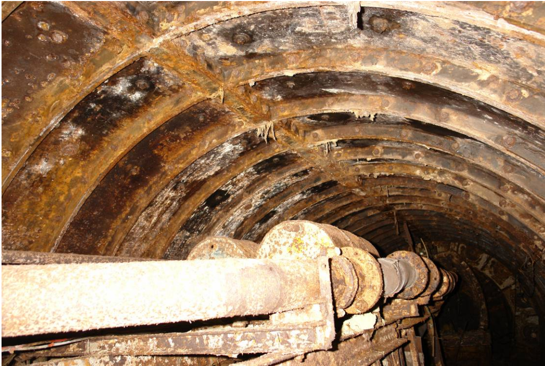
Figure 15 View of tunnel at far end (segment No 250) including part of tunnelling machine
