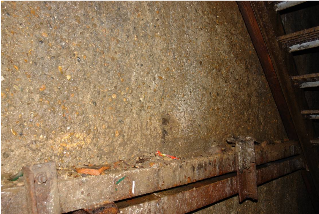
Figure 5 Rough surface finish on shaft walls
