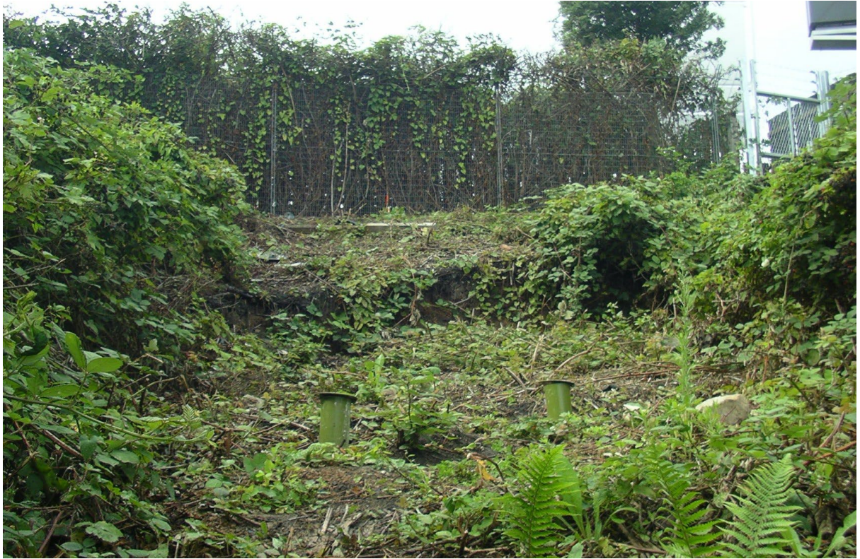
Photo 9.1: Large-scale deep seated failure of a cutting (North Acton)
