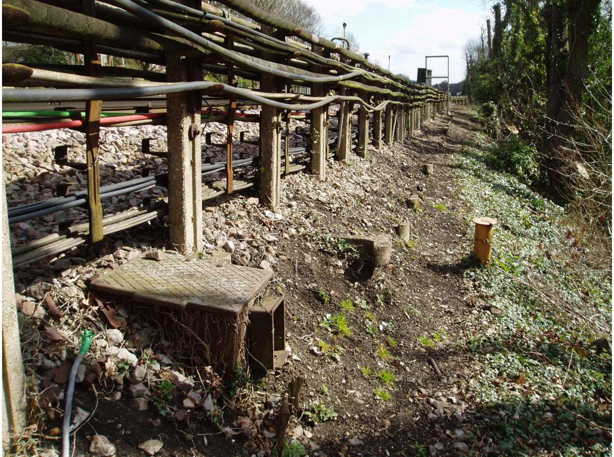
Photo 9.6: Localised crest instability such as raveling ballast should NOT be considered as evidence of instability in the risk classification flowcharts
