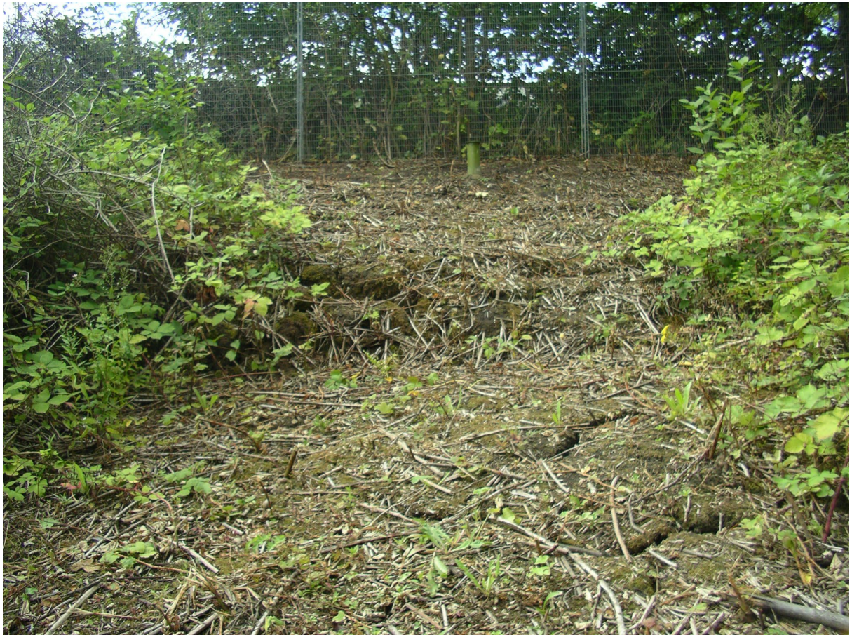
Photo 9.2: Backscar towards the crest of a cutting indicating previous slope failures
