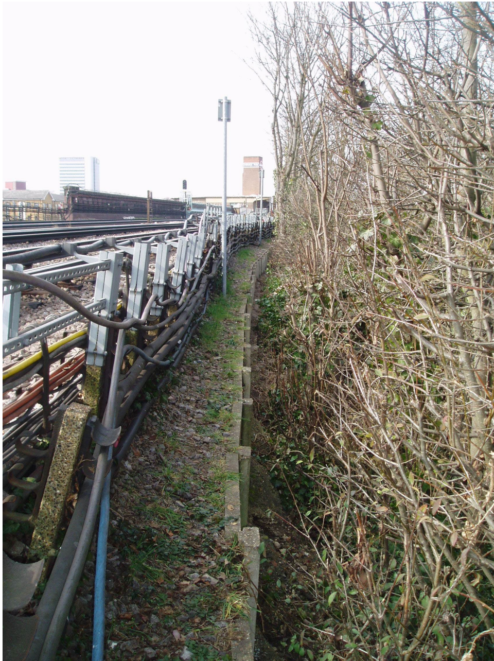
Photo 9.5: Leaning cable posts and vegetation may indicate shallow slope deformation and crest instability
