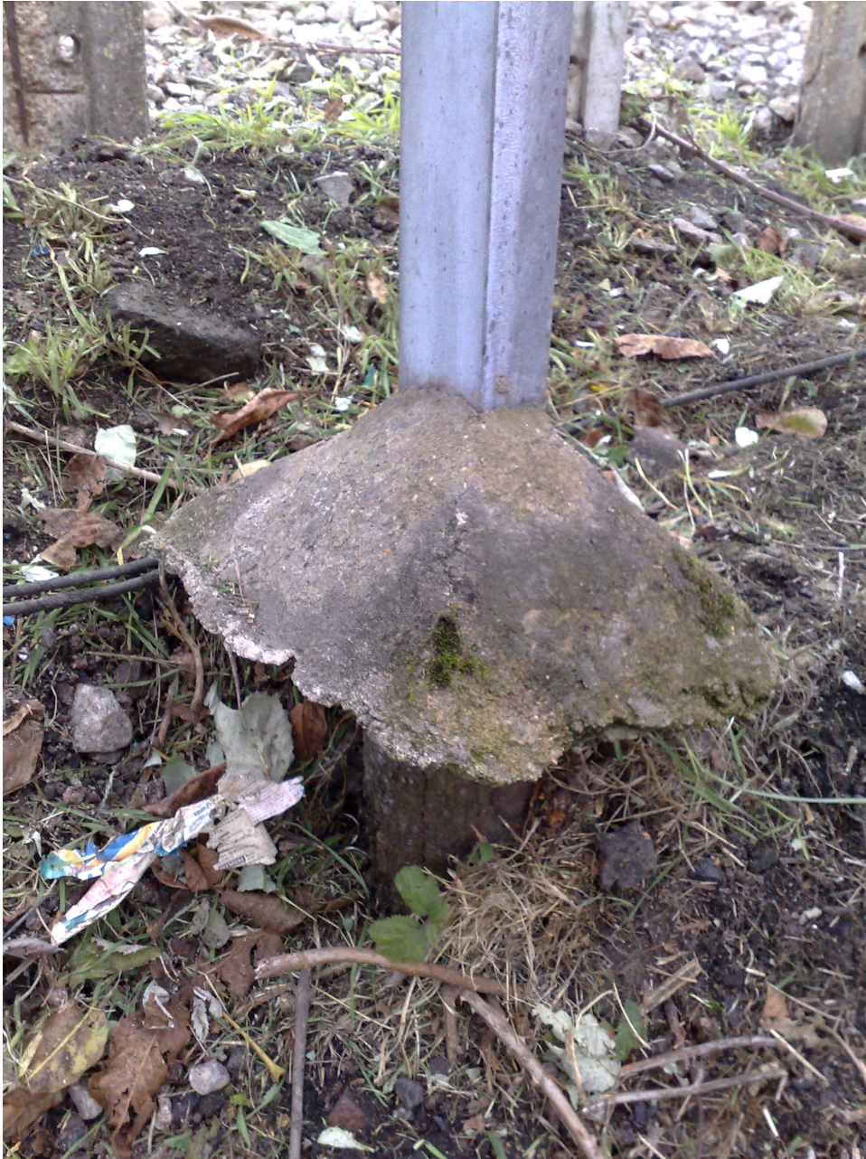
Photo 9.7: Localised slope deformation (NOT related to deep seated instability)
