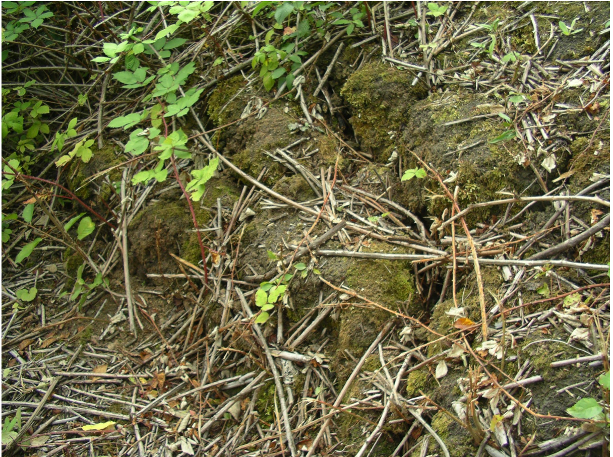
Photo 9.3: Tension cracks at the crest of earth structures may be indicative of deep seated instability
