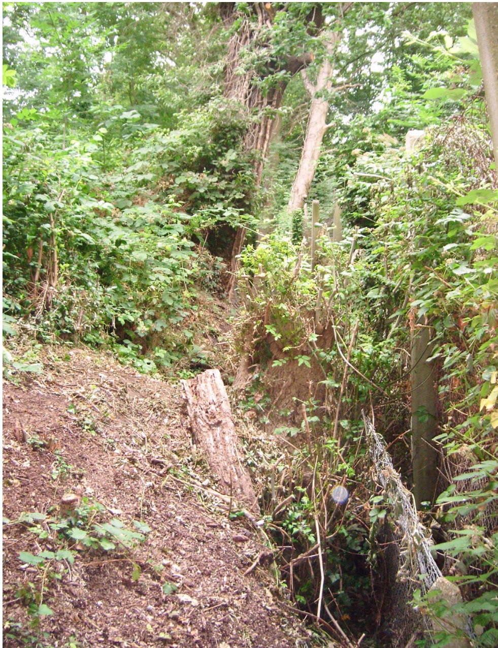
Photo 9.4: Toe bulging may be indicative of deep seated stability
