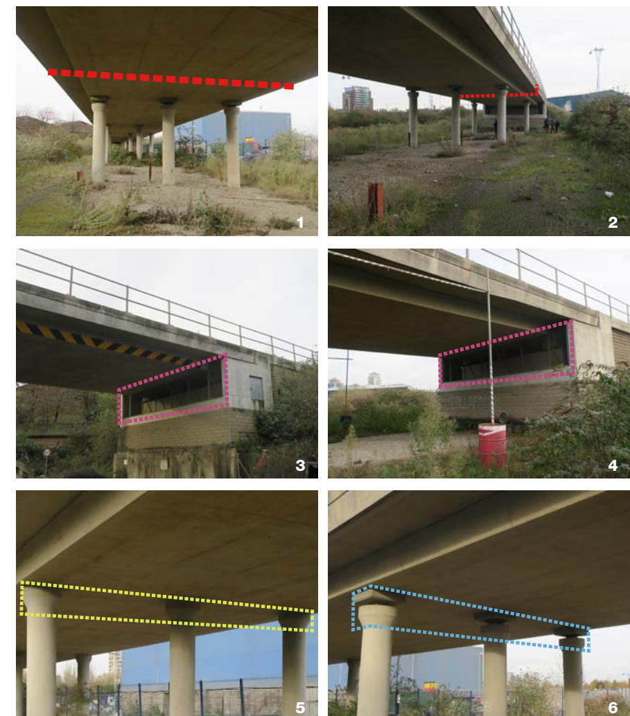
Figure 2a - Site Photographs 1: Space under Viaduct looking to the West 2: Space under Viaduct looking to the East 3: West Abutment 4: East Abutment 5: Integral Columns 6: Columns with Bearings
